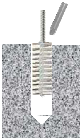
Clean hole by brushing and blowing to remove all dust and drilling debris
